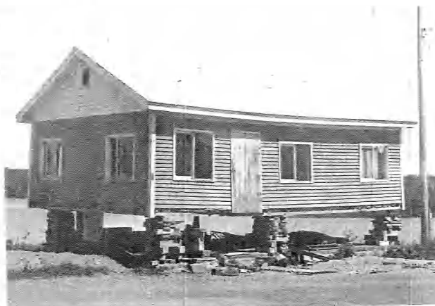
GOING, GOING . . . This home will be moved and saved, but others like it have been demolished at Peter Dana Point, to make way for new housing on the Indian Township Passamaquoddy reservation. The tribe received a $400,000 federal grant to raise 21 houses cited as substandard. Those homes were built a number of years ago by the state, using funds reserved for the tribe.
