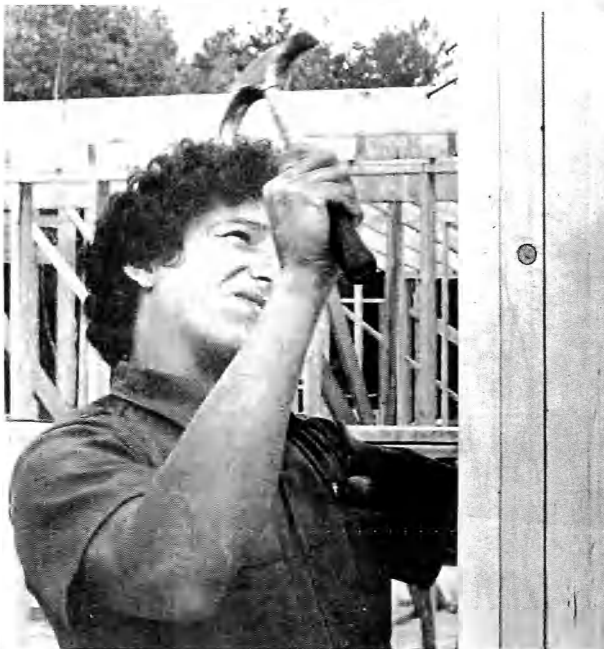
Kevin Mitchell, a Penobscot, works on construction of new medical center at Indian Island. See Health Director story page one. [Cartwright Photo]
